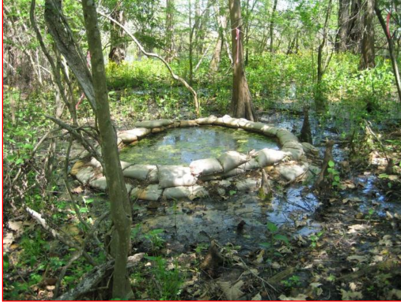
Figure 1.4 Primary levee failure mechanisms: Bagged sand boil near Eagle Lake, MS
