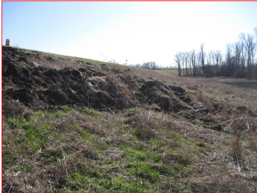
Figure 1.3 Primary levee failure mechanisms: A slough slide on the levee adjacent to Chotard Lake, MS
